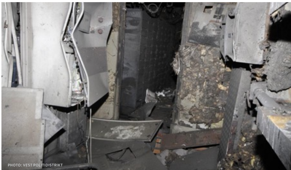
Technical room on board MS Ytterøyningen before the explosion.
