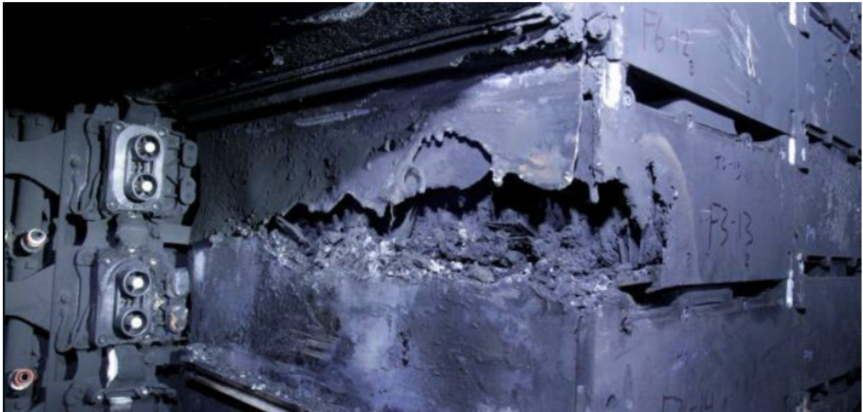
MS Ytterøyningen, the battery fire destroyed the steel casing. Image: National Criminal Investigation Service.
