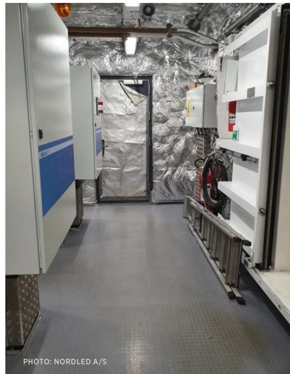
Technical room on board MS Ytterøyningen before the explosion.
