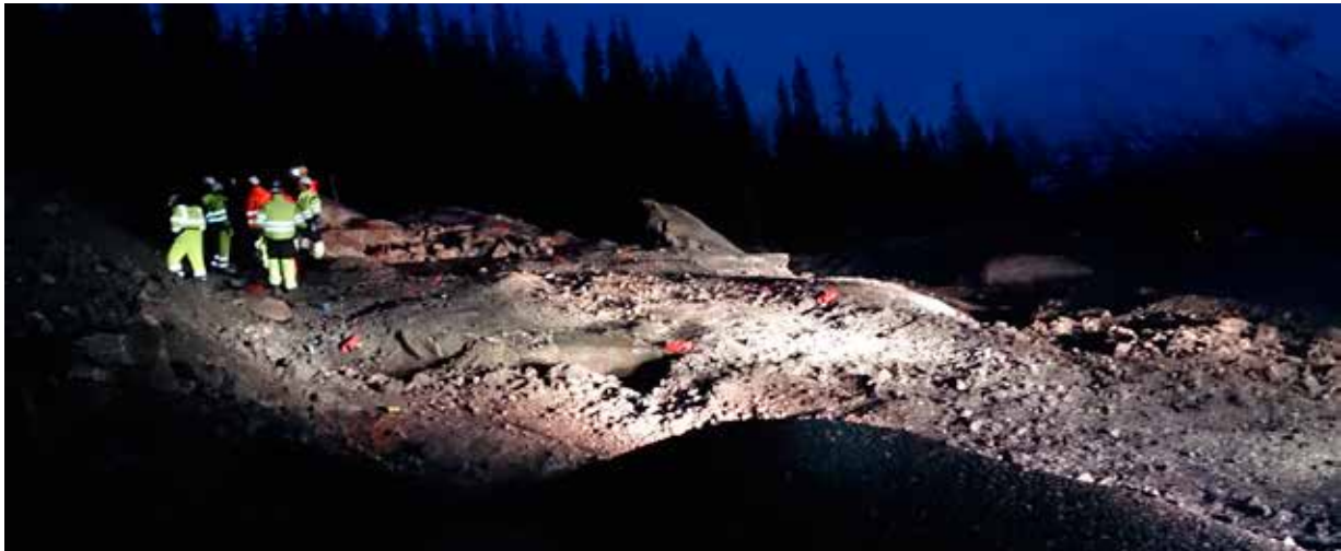
FIGURE 10. Picture that illustrates the effect of the blast on the crushed stones.
