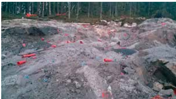
FIGURE 11. What it looked like on the blast area after the explosion.
