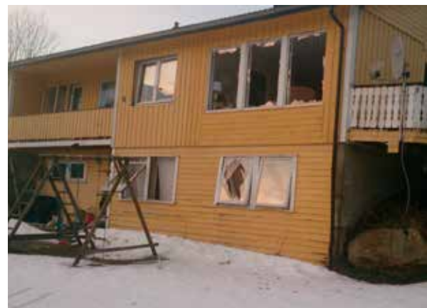
FIGURE 15. Yellow house-wall facing south.
